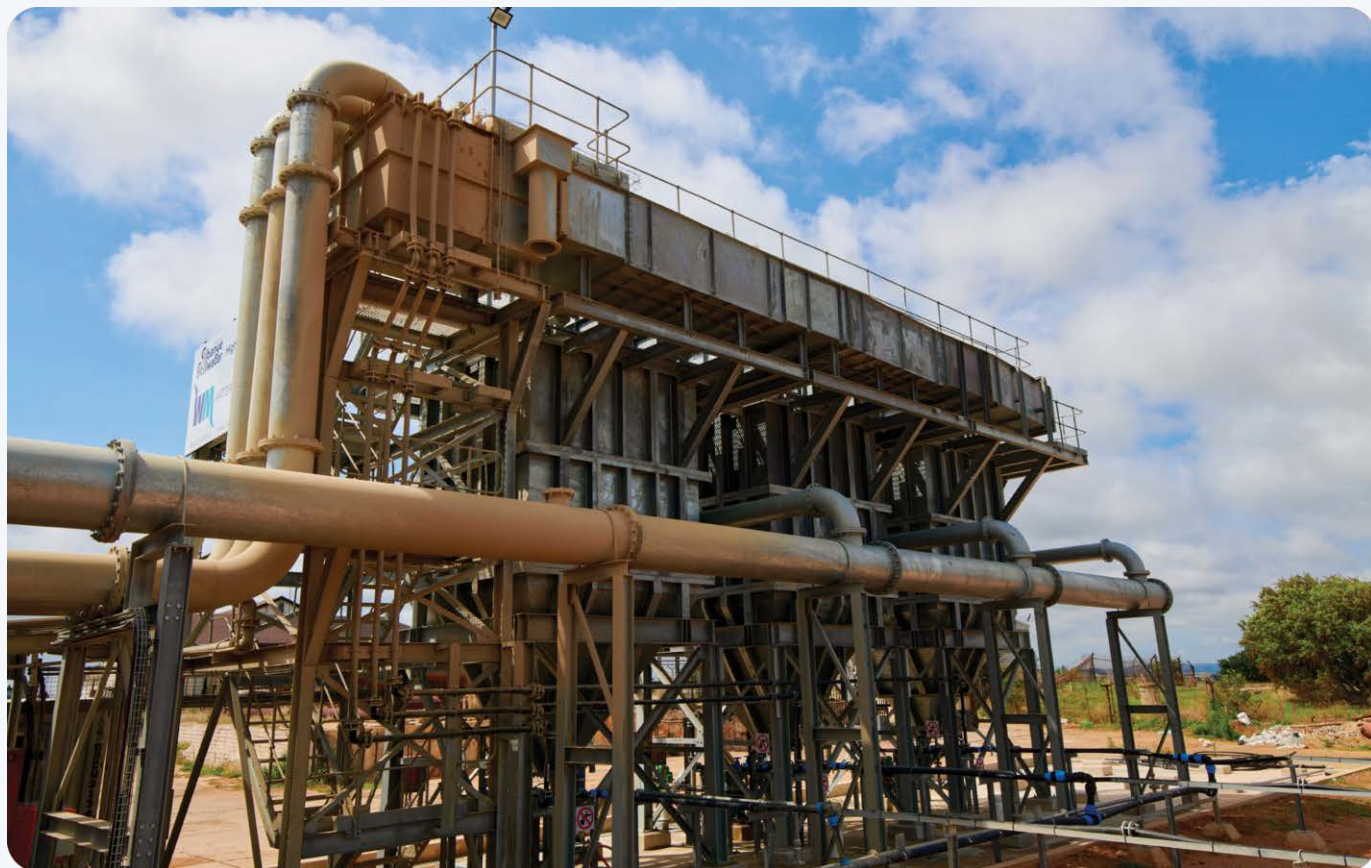
Water treatment plant at the Cooke operation, SA gold operations
