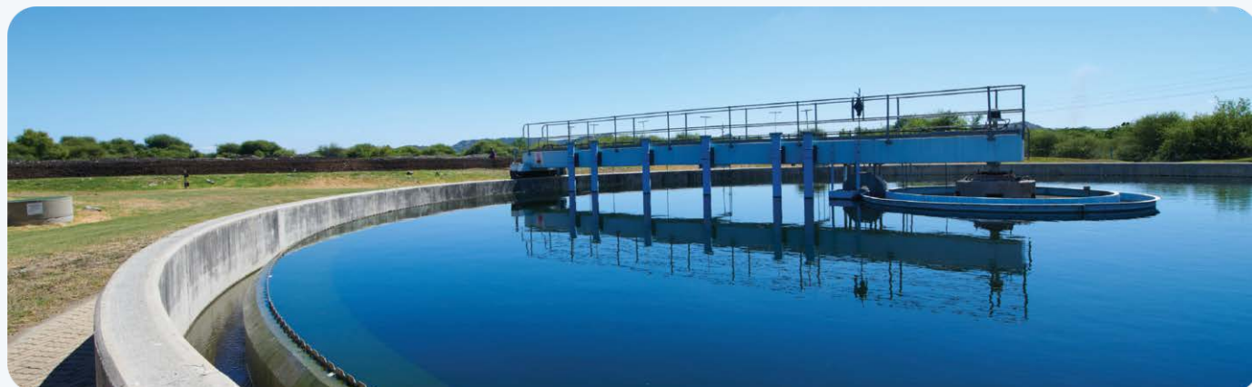
Wastewater treatment plant at Wonderkop, Marikana operation, SA PGM operations
